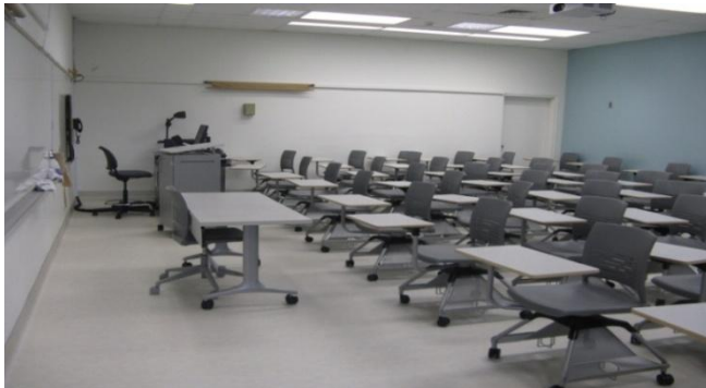
New Sheet Vinyl Flooring
